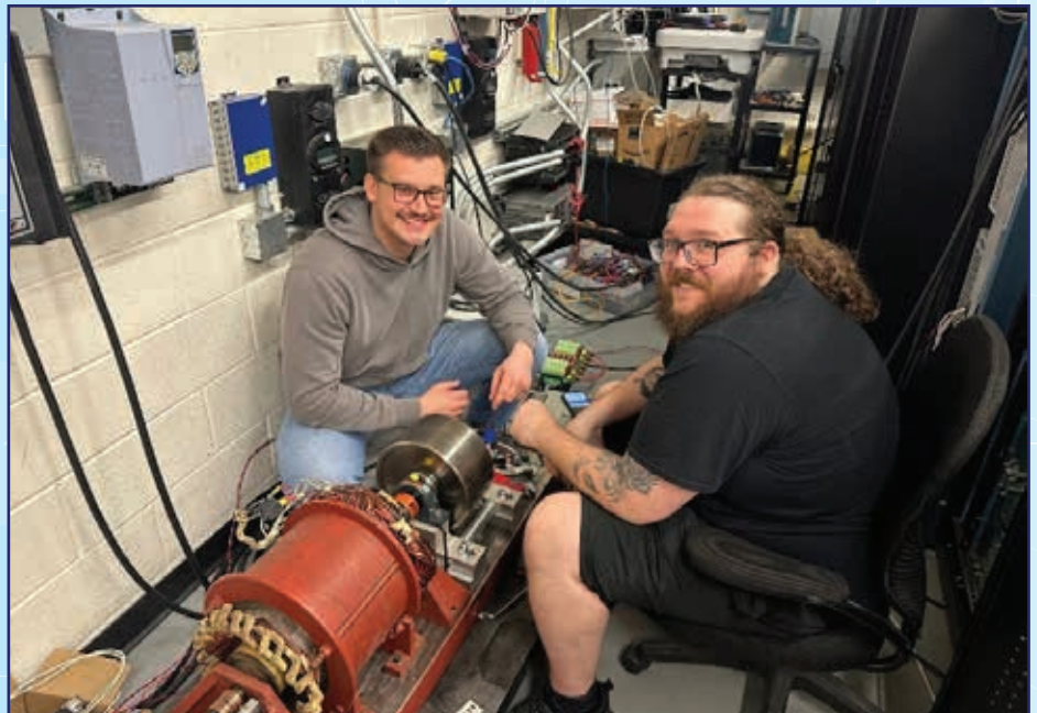
Students work on installing a flywheel energy storage system into motor-generator set.
